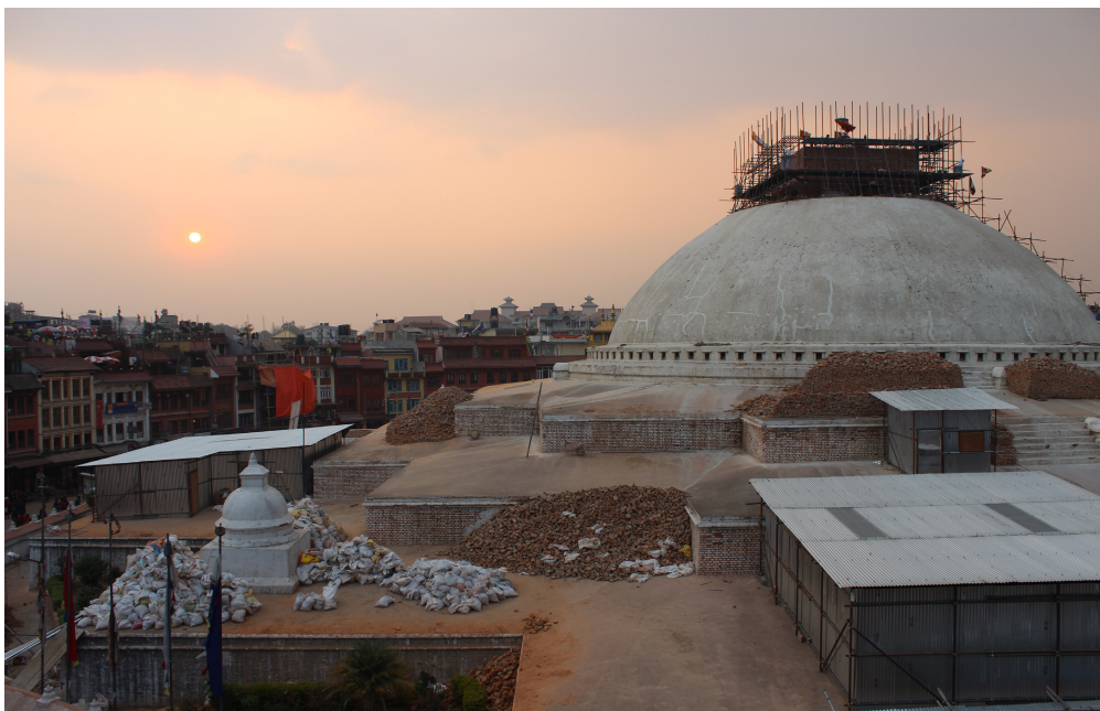
Figure 1. Striving to come back, brick by brick (Photo of Boudha stupa, under scaffolding).
