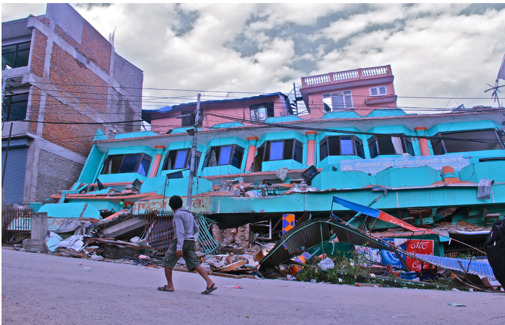
Figure 2. Walking and rubbernecking, a young man surveys a collapsed building in the earthquake's aftermath.
