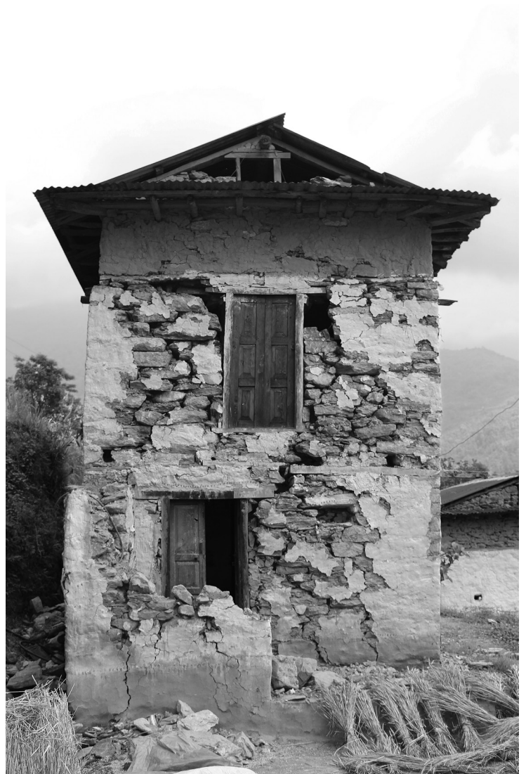
A two-storey stone, mud and wood building that was severely damaged in the May 12 earthquake, Dolakha.
