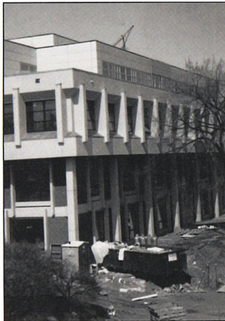
The Humanities wing of the Janet Wallace Fine Arts Center is getting a two-story addition.
