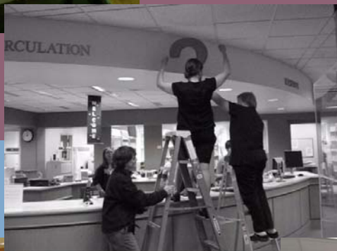
BETH HILLEMANN, ANGI FAIKS, AND TERRI FISHEL INSTALL A COMPLETED QUESTION MARK.
