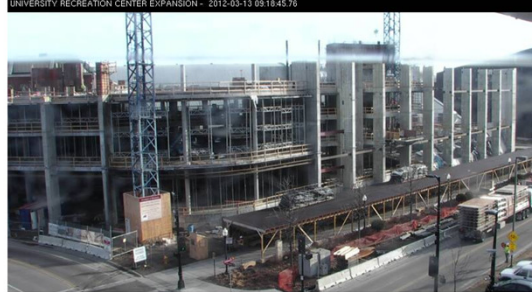
This is a live view of the expansion construction located on the east bank of the University of Minnesota Twin Cities campus.
